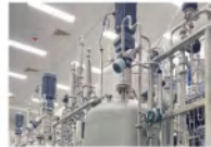
Intelligent pressure regulating valve system
