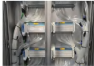
Full intelligent electric and gas circuit control system
