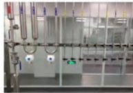
Clean room sewage treatment
