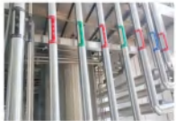
Clean room pipeline through the wall system
