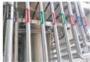
Clean room pipeline through the wall system
