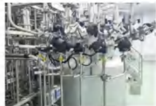
Automatic feeding control system
