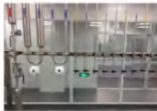
Clean room sewage treatment
